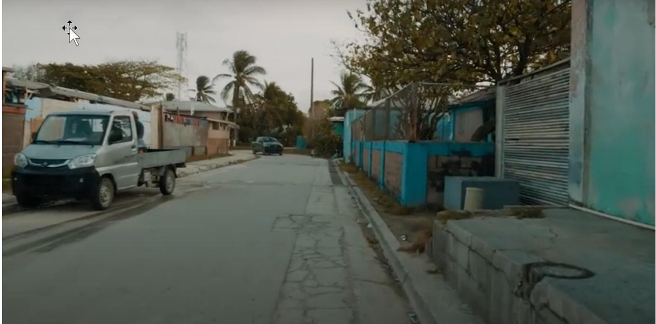
Figure 23 - The more limited space available in Ebeye will make construction more challenging. Hard surfaces will all require reinstatement. Picture shows an example of existing underground infrastructure installation or repair.
