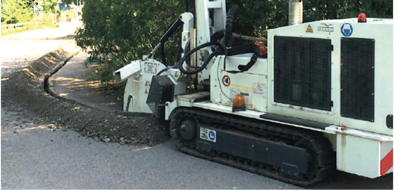
Figure 24- Marais Sidecut SC3C is an example of a microtrenching technology. It can achieve 500m per day in a wide range of terrain. 200km of fibre optics has been deployed in New Zealand by Marais to date. This equipment would be suitable for both Majuro and Ebeye environments.
