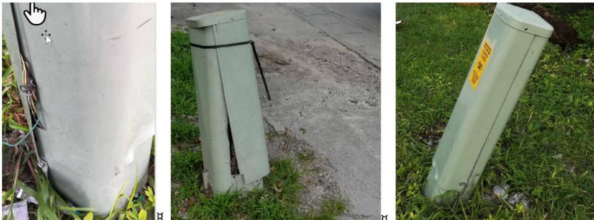
Figure 10 - Examples of Copper network condition in Majuro
