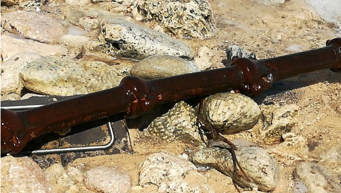
Figure 21 - Articulated Pipes at the landing, showing high erosion and cable in suspension
