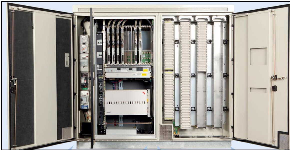
Figure 8 - Example of powered telecommunications cabinet with battery backup that would provide for the Larua needs compared to the existing Shelter and associated infrastructure. Fiber equipment is on the left, cable termination on the right.
