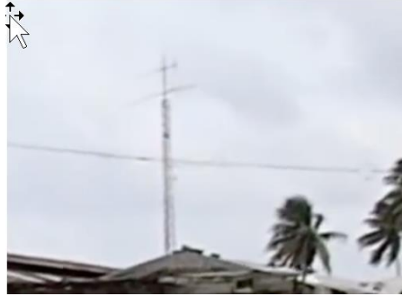
Figure 18 - HF Radio antenna on Majuro
