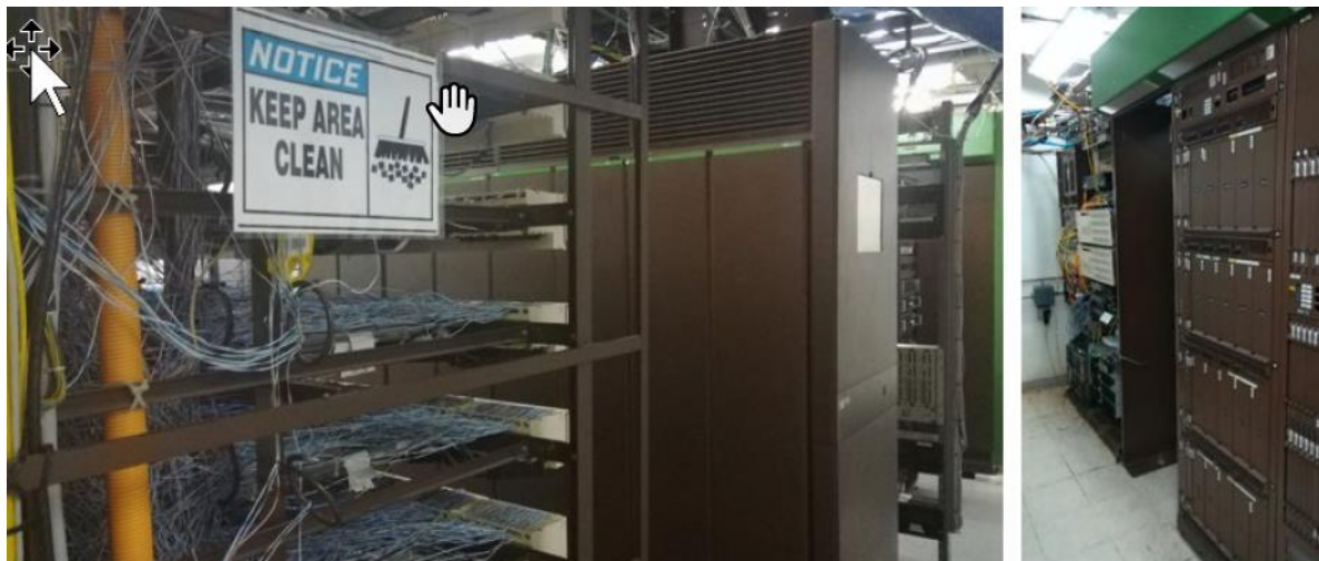
Figure 14 - Existing Nortel telephone exchange and equipment. The left is the copper termination in the main NTA building, the right is an example of the equipment in the remote sites of Airport and Laura.
